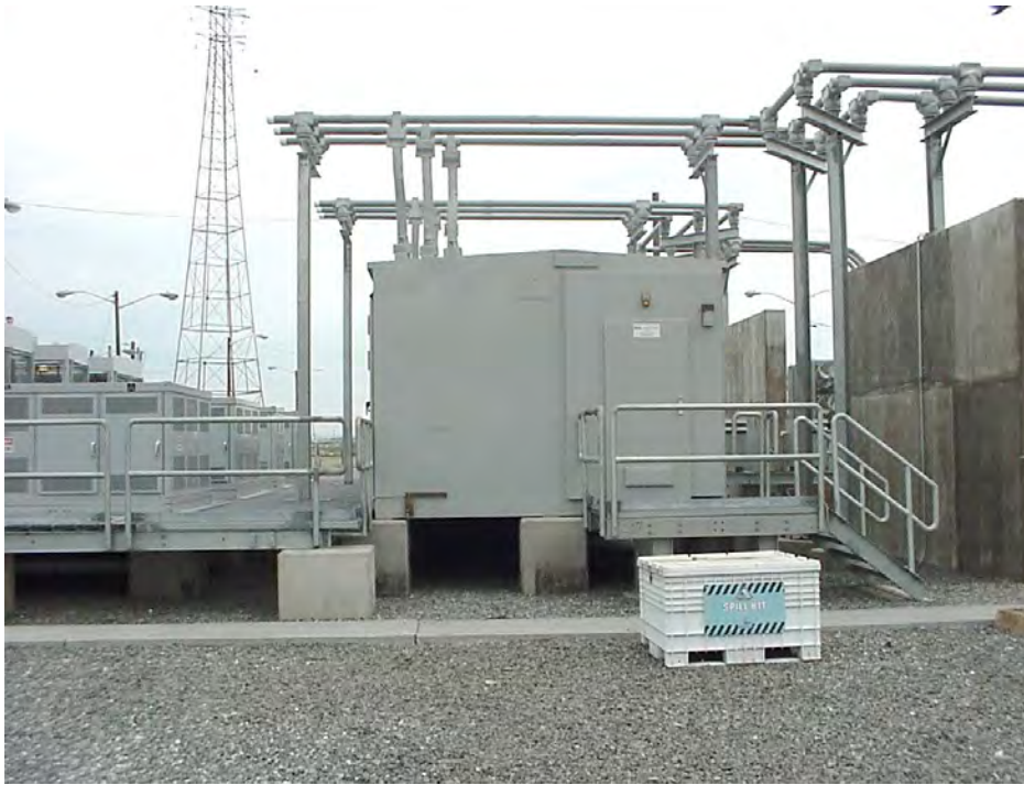
Figure 6 - Metal Enclosed 4 kV Switchgear [Outside View]
